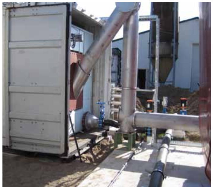
External view of a hydrogen reactor: at least 10% higher energy yield.
