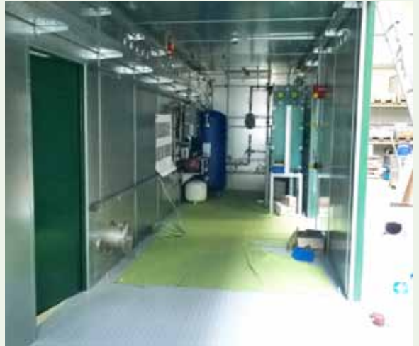
Just two weeks after the delivery of the containers, the first construction phase has been completed: the cold water storage unit and heat exchanger are installed inside the machine container.
