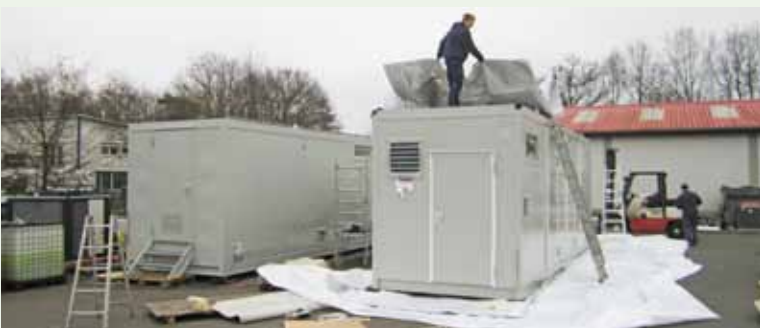
It is finished. After a total of 1300 working hours, both containers are ready to be transported to the Chinese customer on the 9th of December 2014. Before loading, both containers must be packed carefully.
