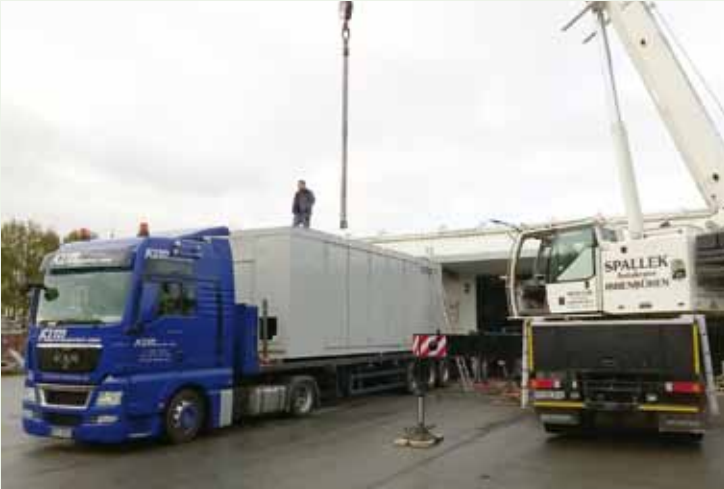
At the beginning of November, the two machine and membrane containers are delivered by lorries and heavy-duty cranes to the EnviTec production location in Saerbeck. The interior fittings can now be started!
