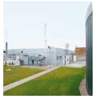
Commissioned in 2013: the two EnviThan gas upgrading plants at Sachsen- dorf (top) and Köckte.
