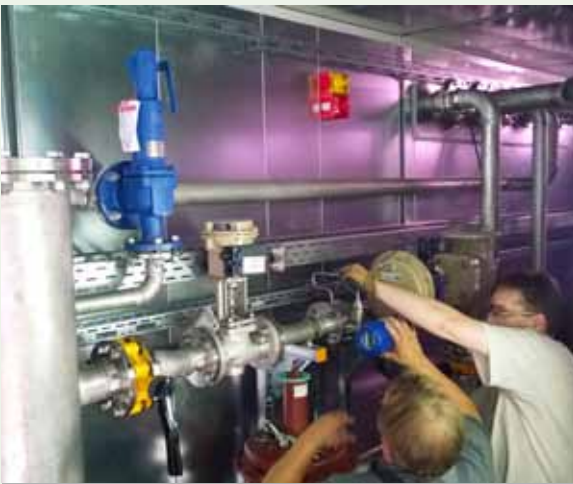
Who wants to see hard-working workmen? A total of nine technicians assemble the container unit in Saerbeck. Armatures and valves are installed by the technical experts.
