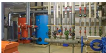
The heat arrives in the cellar of the home and is distributed throughout the building.
