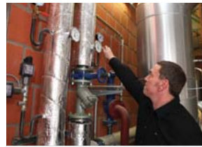
The plant supplies heat in the form of hot water and saturated vapour.
