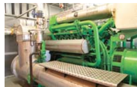
The heat comes from the biogas plant's co-generation unit.
